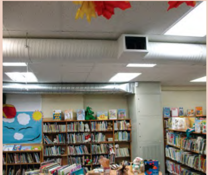
Installed flat-oval ductwork is shown in one of the school's classrooms.
